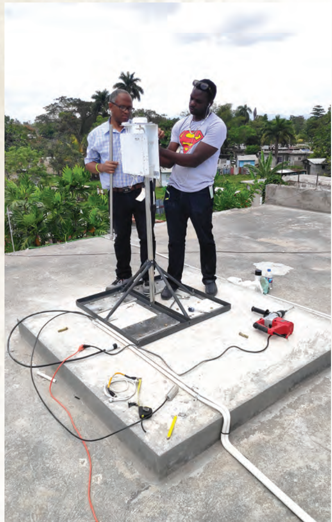
Figure 9 - Mr. Philmore Trowers, Manager Monitoring & Inspection with a Technician, facilitating the installation of new equipment at the new Savannah-La-Mar monitoring site.
